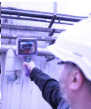
COMPRESSED AIR LEAK DETECTION
